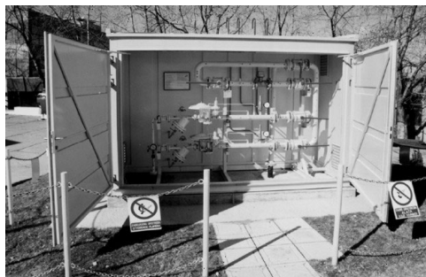
Merno-regulaciona gasna stanica
